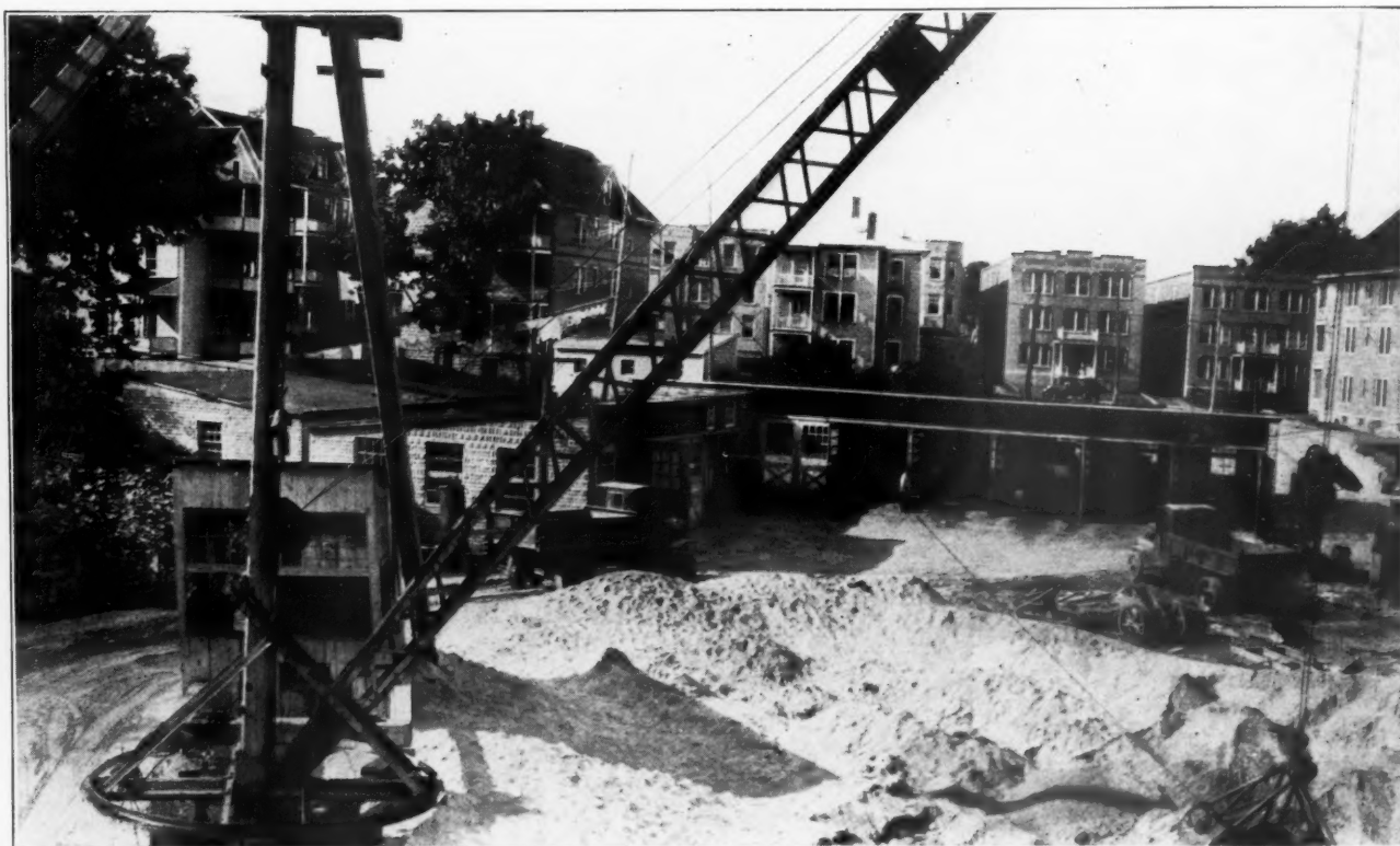
View from Top of Screen House, showing Derrick, Stock Sand Pile and Garage
